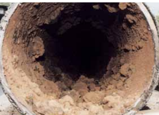
Heavily encrusted steel pipe
