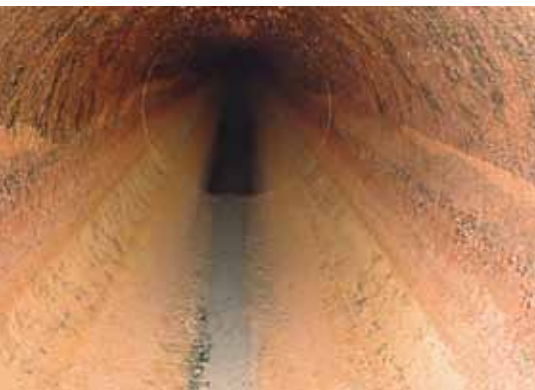
Heavily corroded steel pipe
