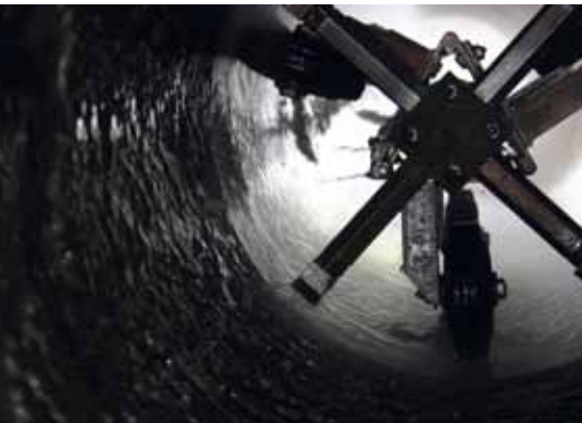
Cleaning the old pipe with the maximum water pressure up to 2400 bar
