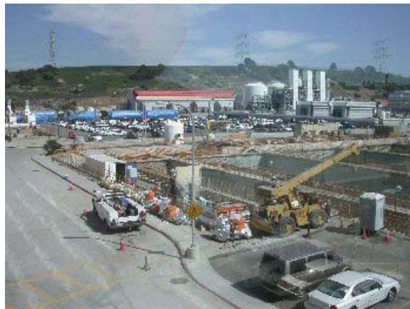
Figure 1. Hyperion Treatment Plant Emergency Bypass Channel
