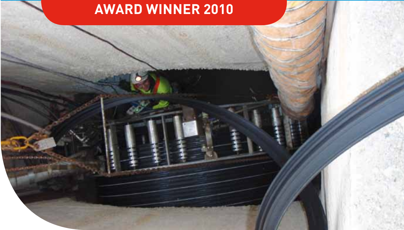
Winding the 2400mm diameter SPR™ PE pipe from inside the access chamber.
