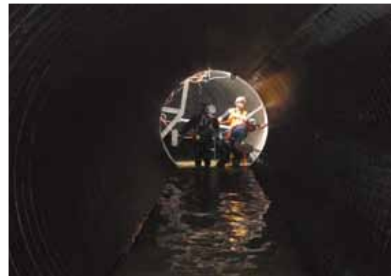
The sewer had to remain operational at all times so work was performed in live flow.
